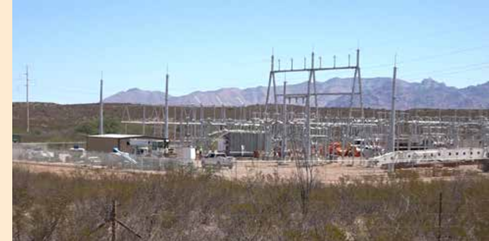
Schieffelin Substation can be seen east of Highway 80, north of Tombstone.
