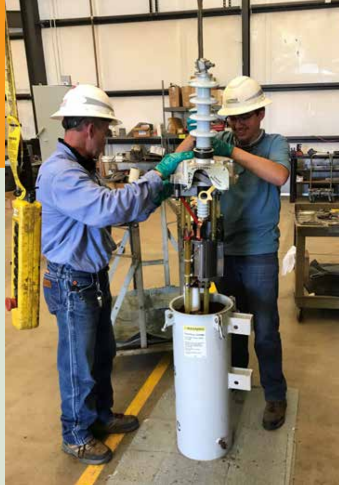
Bill Roethle teaches intern Mark Smalling the internal workings, purpose and operation of single phase reclosers.
