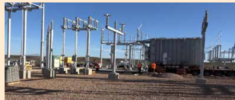
The transformer had to be delivered and placed via the "jack and move" method because the substation was too narrow to accommodate a crane delivery.
