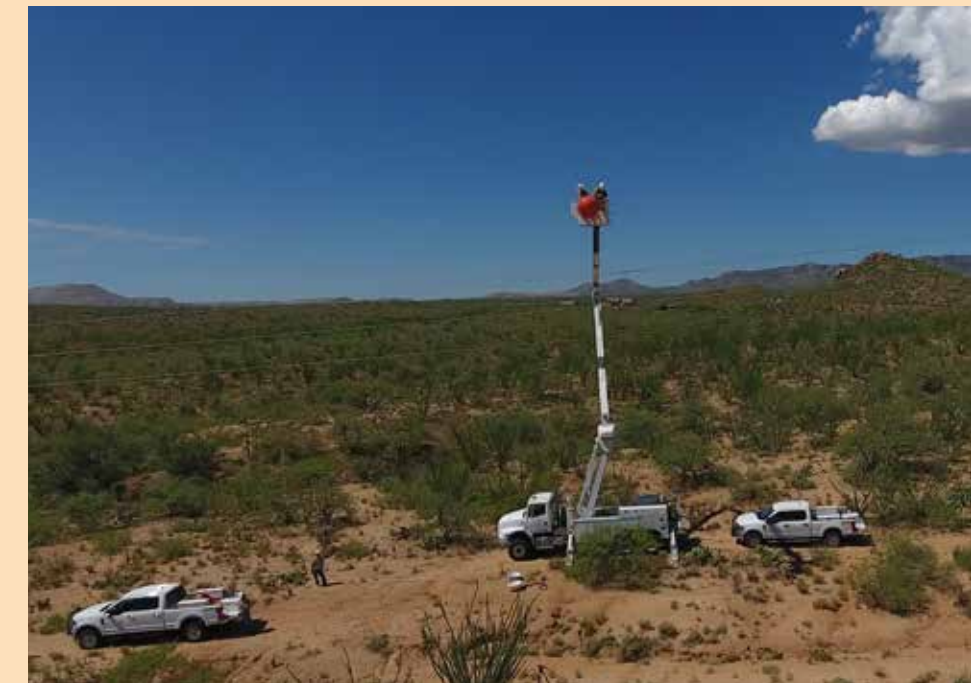
This is an aerial view of the AzGT line crew replacing transmission line visibility markers on the 115 kV Bicknell-Three Points line. Tony Ferraro, hotstick lineman, and Brandon Guinane, hotstick lineman apprentice, are in the bucket.
