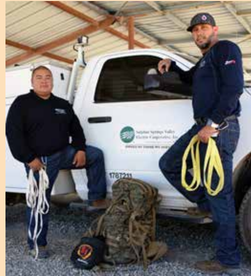
Rafel Villegas, left, and Adrian Fuentes, right, used straps and ropes to carry a 75-pound air conditioning unit, and a 100-pound pack of tools, to the top of Dos Cabezas to make repairs to communications equipment.
