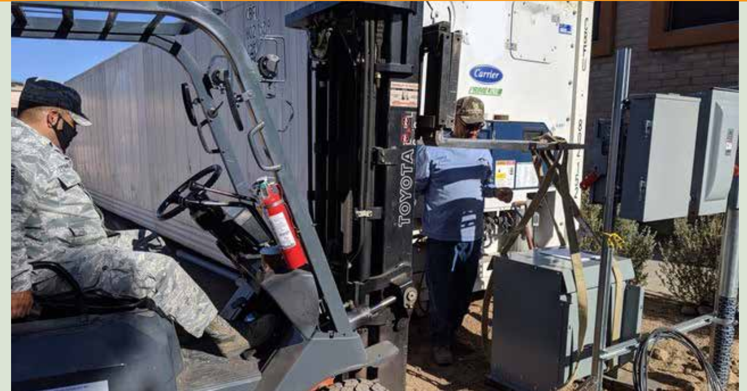
Trico lineman Jaime Esparza (right) directs Omar Fernandez where to place a transformer for the container.
