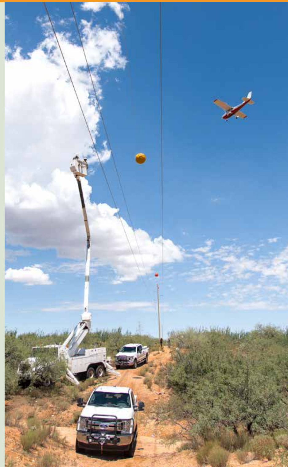
A private plane comes in for a landing at the Flying Diamond Airpark west of Sahuarita, as the AzGT line crew replaces transmission line visibility markers on the 115 kV Bicknell-Three Points line.
