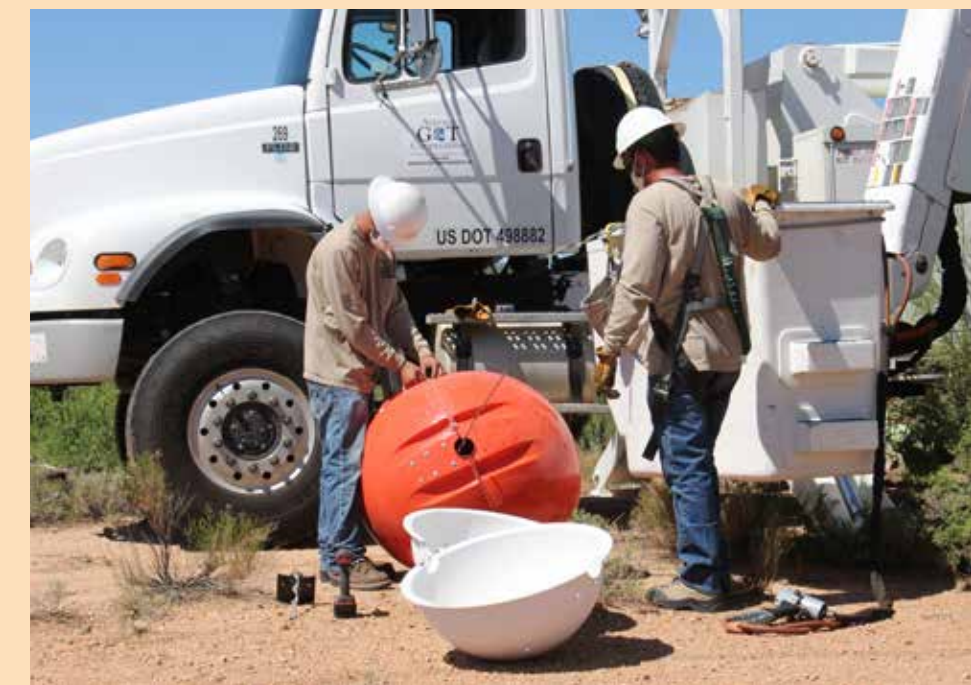
Brandon Guinane (l), hotstick lineman apprentice, and Tony Ferraro, hotstick lineman, assemble a new transmission line visibility marker (orange ball) before installing it on the 115 kV Bicknell-Three Points line. The white ball is the old marker that was being replaced.
