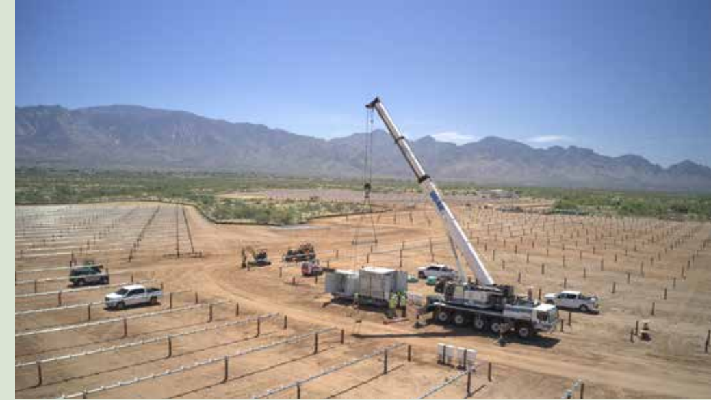
A crane moves the Tesla batteries at the Chirreon Solar and Battery Facility to prepare for the installation of solar panels.
