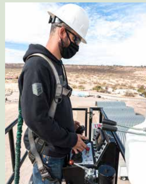
Jordan Tracey operates the bucket as the boom is fully extended to a height of 150 feet.
