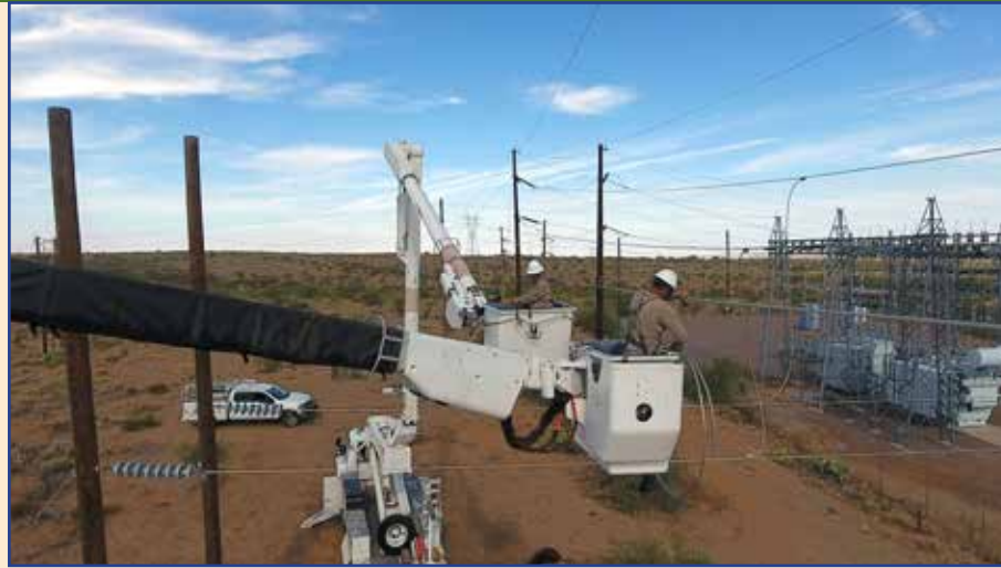
This aerial (drone) image shows Tony Ferraro (foreground) and Brandon Guinane in the buckets as they work to install bypass conduit at the Oracle Junction substation.
