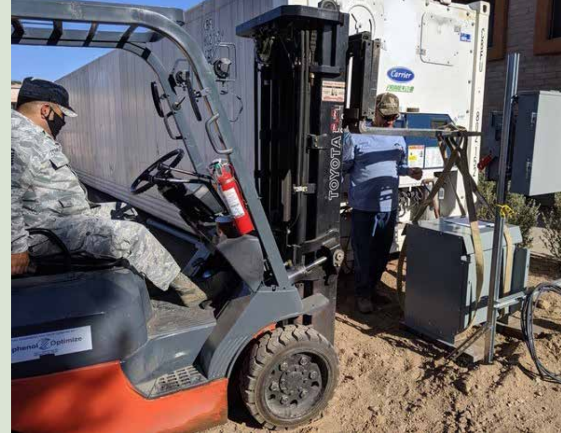
Trico Electric Cooperative's Jaime Esparza and Master Sgt. Omar Fernandez (l) install a transformer at the Sahuarita Food Bank. (Photo Courtesy: Trico EC)
