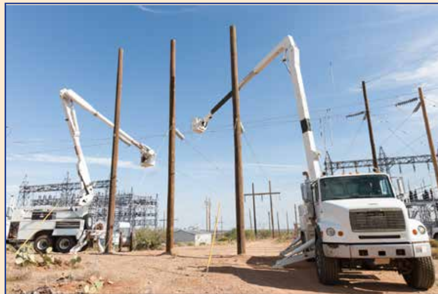
This image shows the "shoe-fly," an industry term or slang for a temporary structure used to bypass a substation. This "shoe-fly" consists of three poles on each side of the substation complex and the conduit that was installed for a project in 2014.
