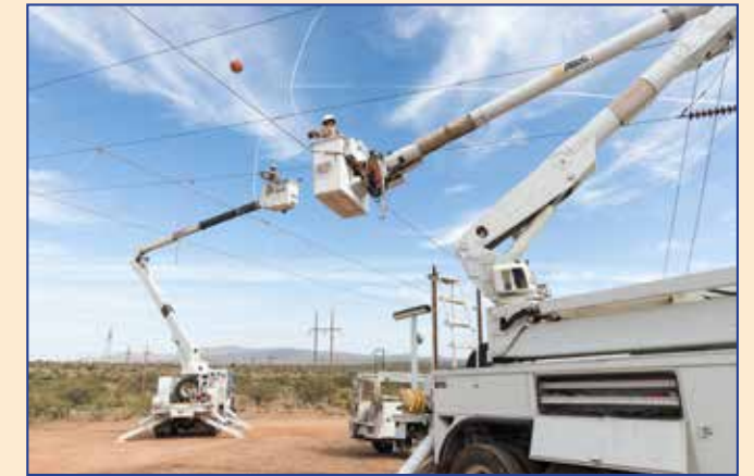
This image shows the view from below as Tony Ferraro and Brandon Guinane maneuver the booms to get access to the bypass conduit on the "shoe-fly."
